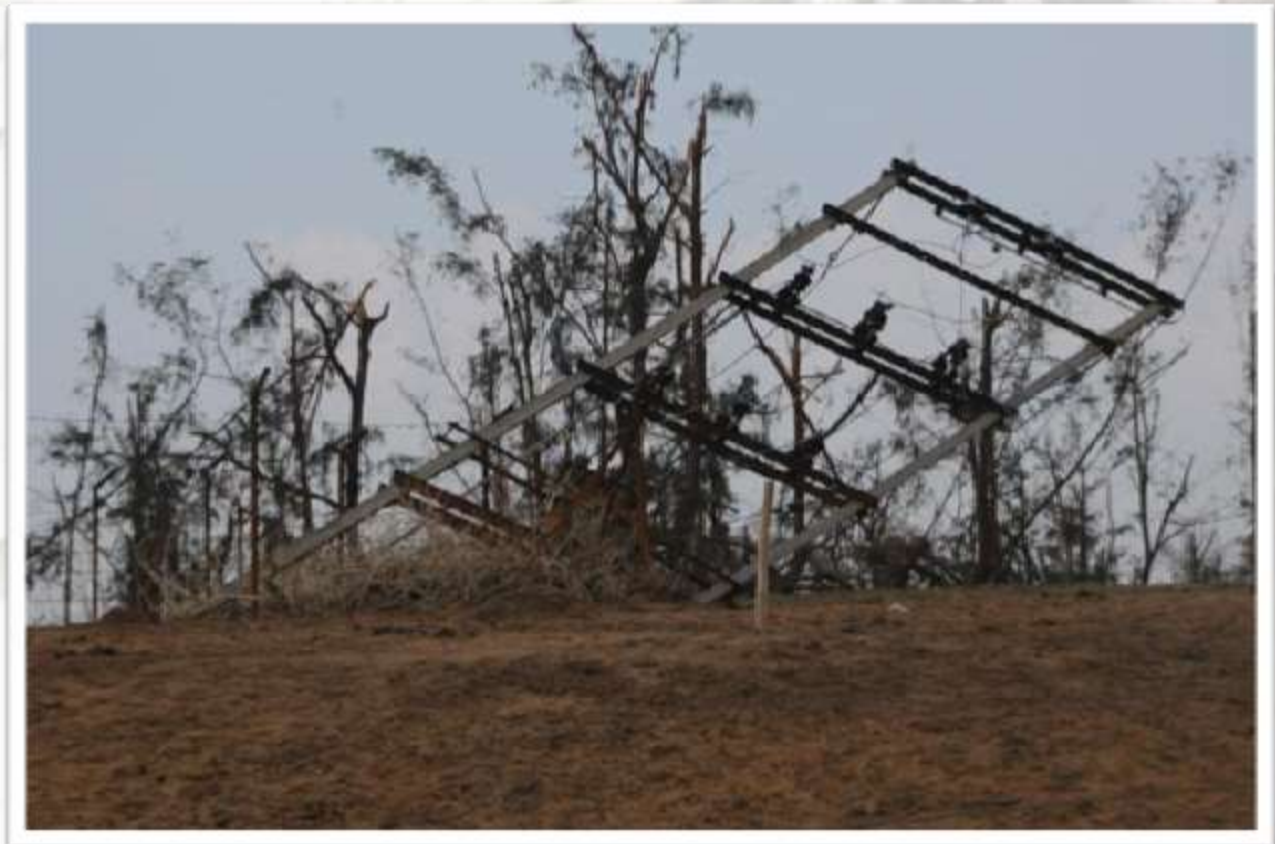
(A mangled electrical transmission tower is pictured after Cyclone Phailin made landfall in Berhampur)
